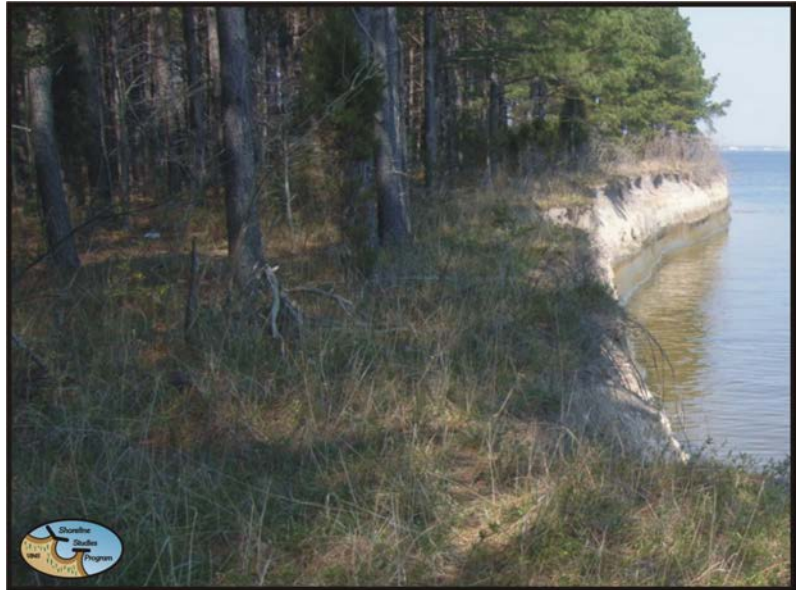
Figure 3-1. One example of forest management. The edge of the bank is kept free of tree and shrub growth to reduce bank loss from tree fall.
