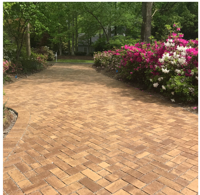
The completed driveway replacement. The landowners report that their previous driveway runoff issues have been resolved with this practice.
